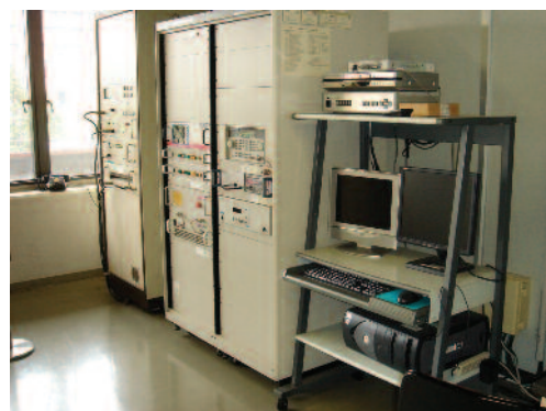
Figure 4 Control system of the renovated electromagnetic environment test facility (NMIJ)
